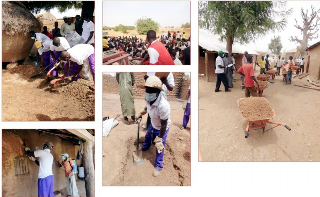
Figure 6: Remediation in Affected Communities
